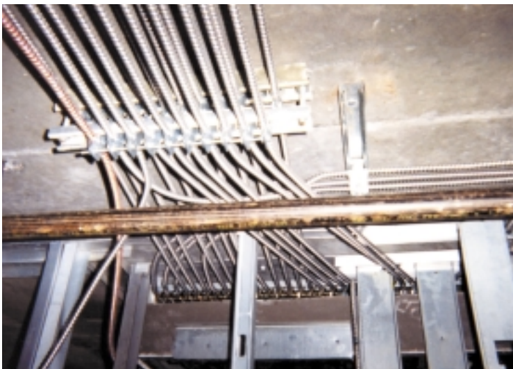
Electricians ran the pre-wired MC cable through existing holes in the metal stud work.
