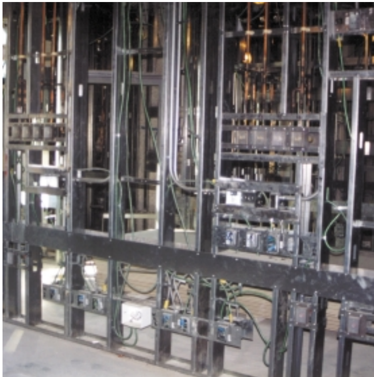
Contractors reduced wiring time by installing HCF-90 in place of pipe and wire.
