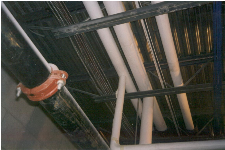
Fully plenum rated, FACC was fished above plaster ceilings at the Fairhaven High School in Massachusetts.
